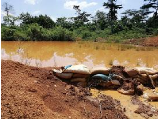
Figure 1a. A leaking tailings dam where the polluted water to flow into upstream rivers.
